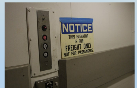
Where there's a will, there's a way.... For over a month, the freight elevator has been out of order. No big deal unless your having to transport food and supplies from the basement to the kitchen, right? They didn't let this slow them down; staff hauled everything they needed up the hill to the kitchen using backbone and a dolly.
