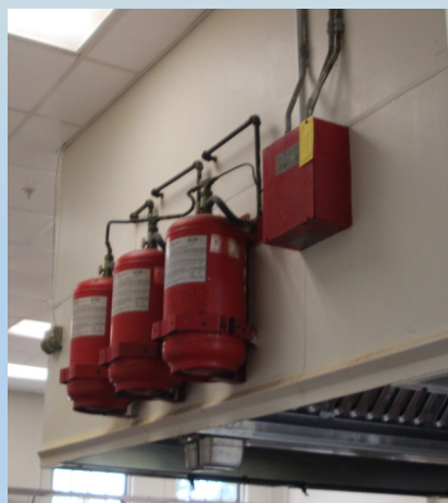
These aren't your typical home fire extinguishers. This hood suppression system and other extinguishers are all up to code.
